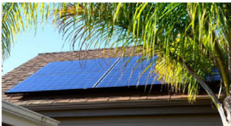
Solar panels on a resident rooftop
