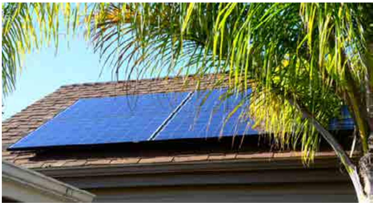
Solar panels on a resident rooftop
