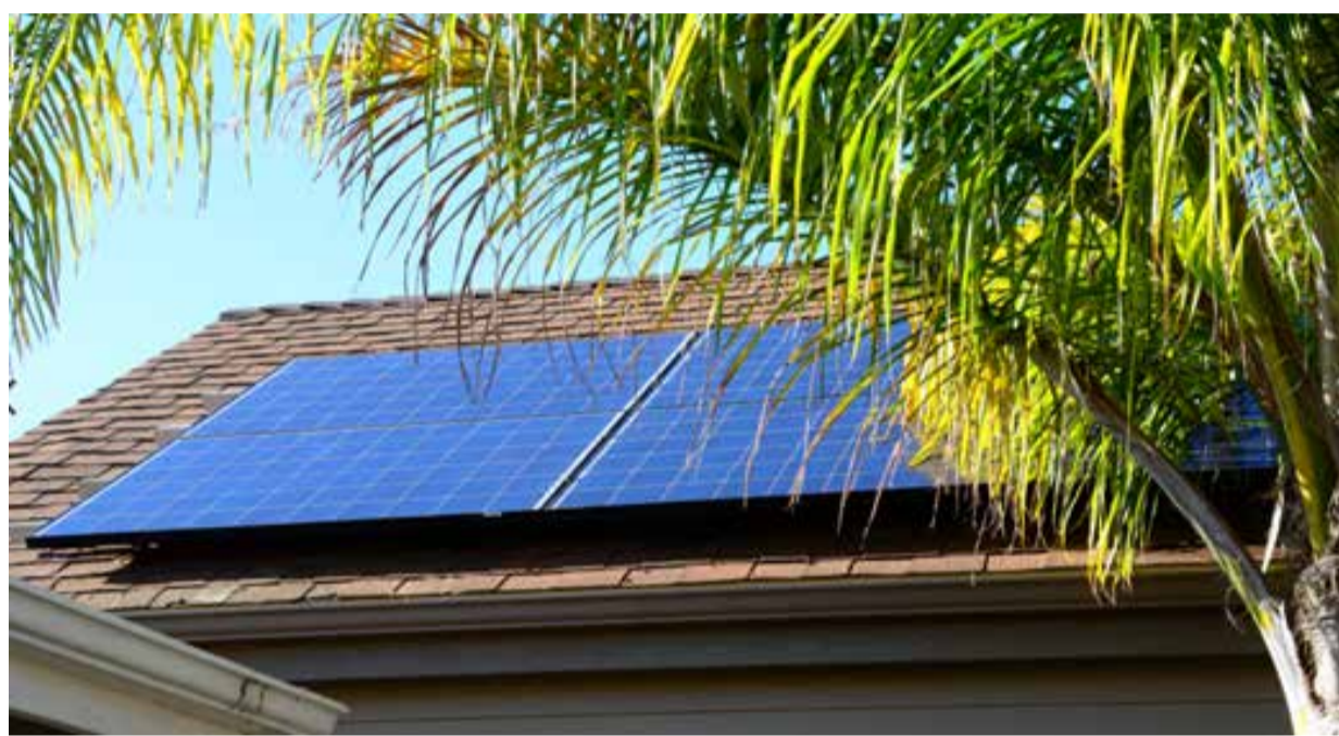
Solar panels on a resident rooftop
